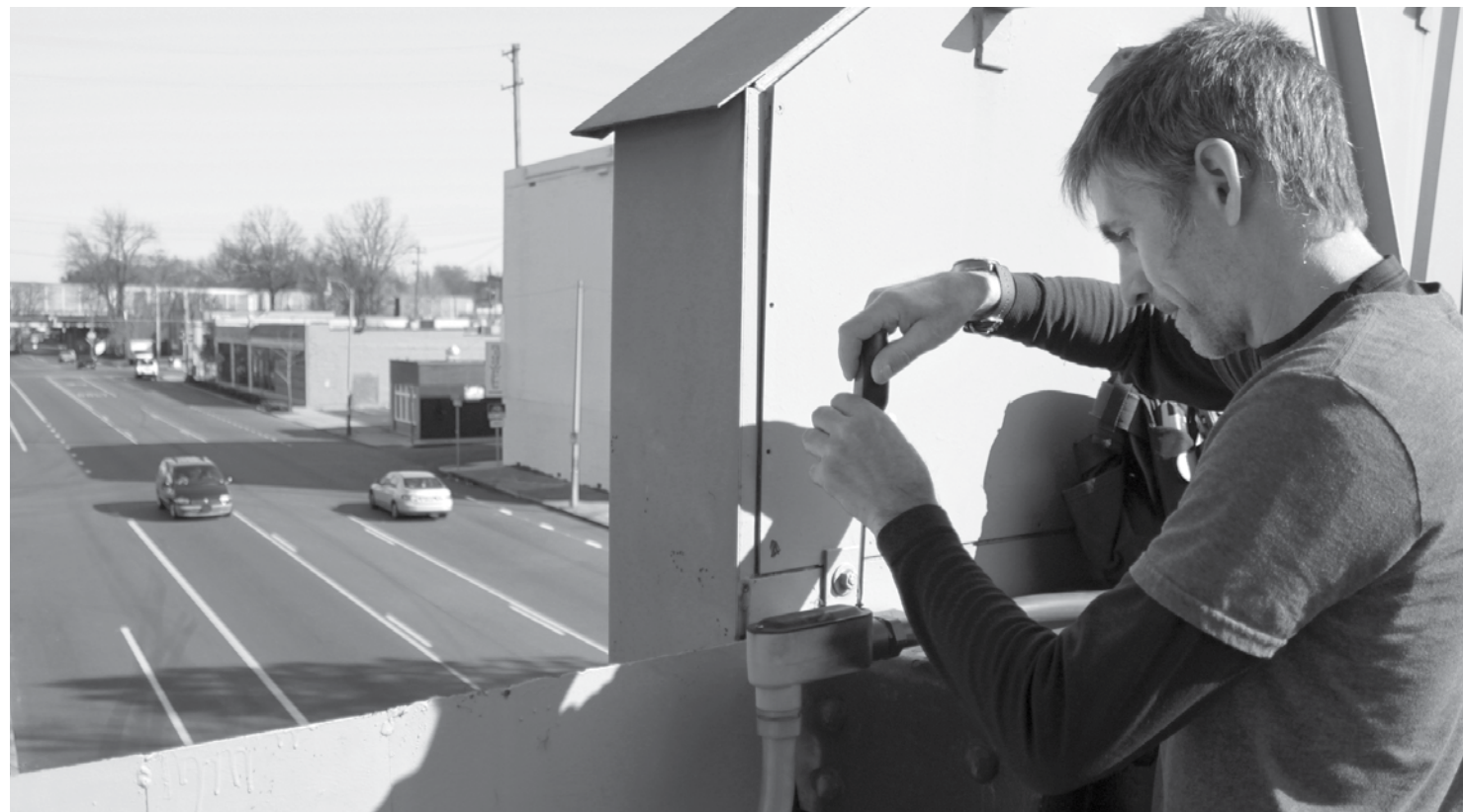
Daurie Schwartz with Schwartz Electric checks the wiring on the Cooper Street trestle art after LED bulbs were installed on Cooper-Young's signature sculpture. The neighborhood is raising funds for the second phase of a project that will install solar panels to generate electricity for the display. Photo by Daniel Scruggs/scruggscreative.com.
